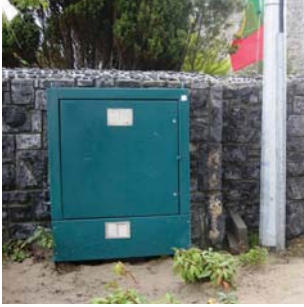
District Regulating Installation (DRI)
