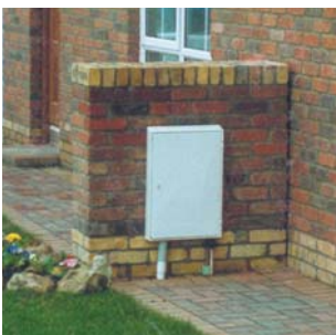
Domestic meter box
