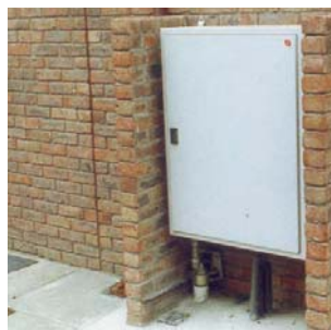
Six meter cabinet
